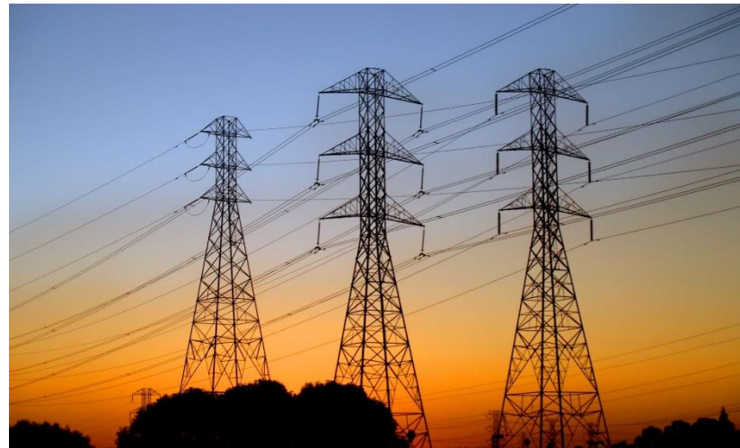
High Voltage Overhead Lines (OHL)
