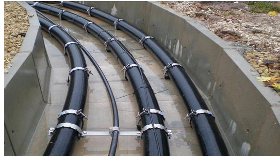
High Voltage Power Cables
